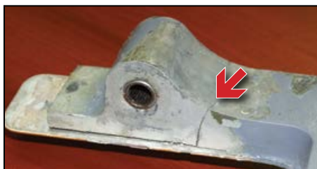
Original hinge showing stress fracture and cracking, separating casting from door skin.
